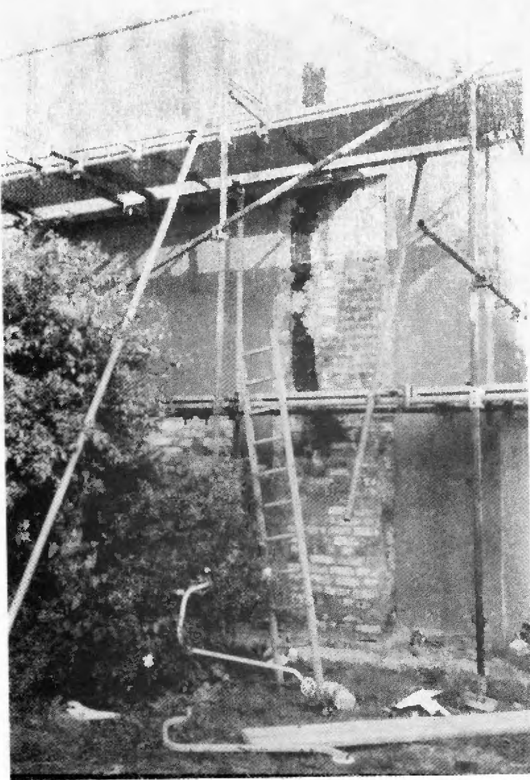
Alterations - a chimney has been removed and the roof raised at the west side
