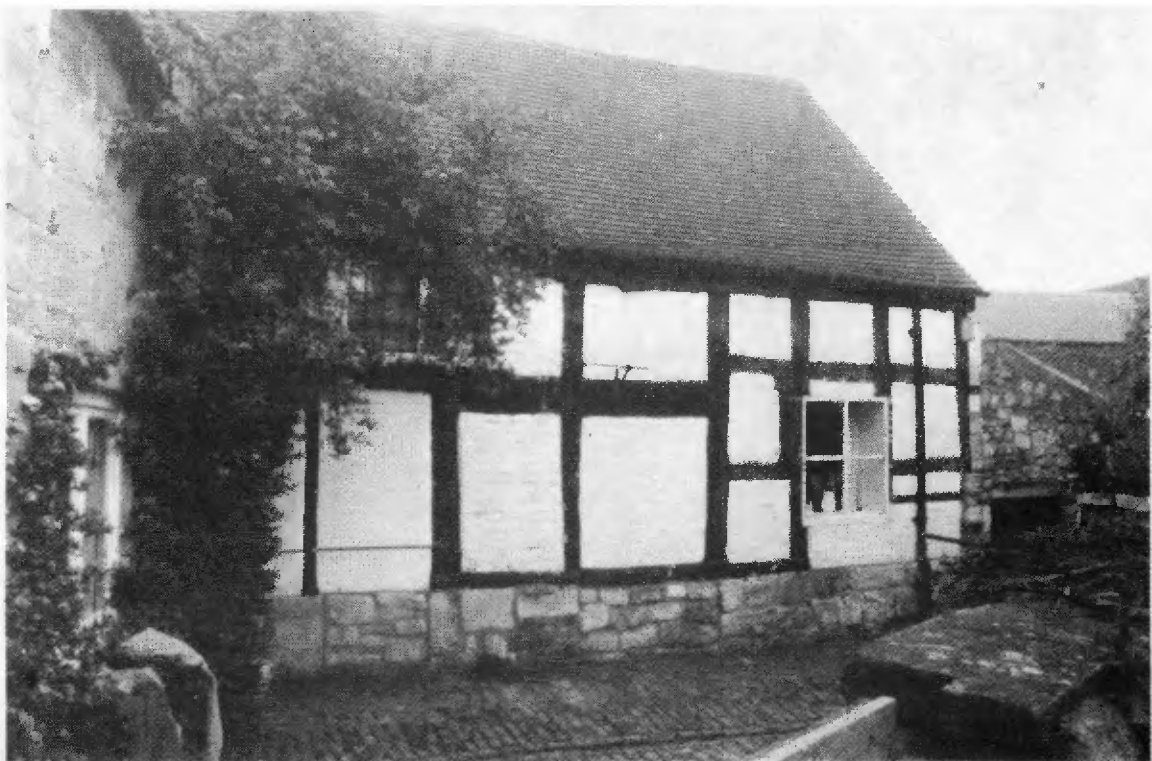
South side of kitchen and cottage (lately used as dairy) - Note blocked doorway.
