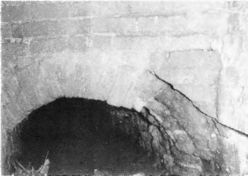
Continuation 1970 as it dropped down to 3 foot - bricks had fallen away on right - This was the older part of the culvert and bridge.
