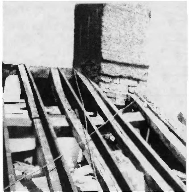
Second chimney inserted at east end of the house perhaps in the 18th century. Note turned timbers.
