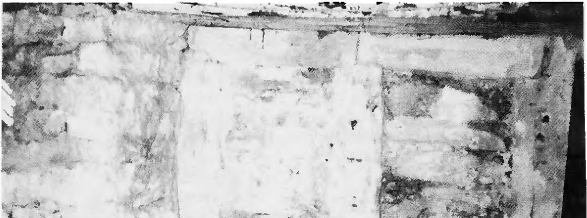
blocked window in cellar
