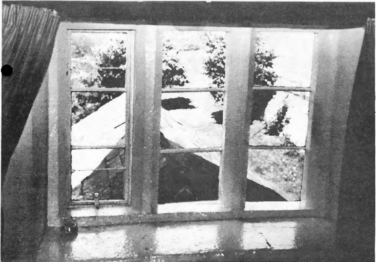
Window in attic (2nd floor) room of rear wing, looking over cheeseroom roof. (L.H.)
