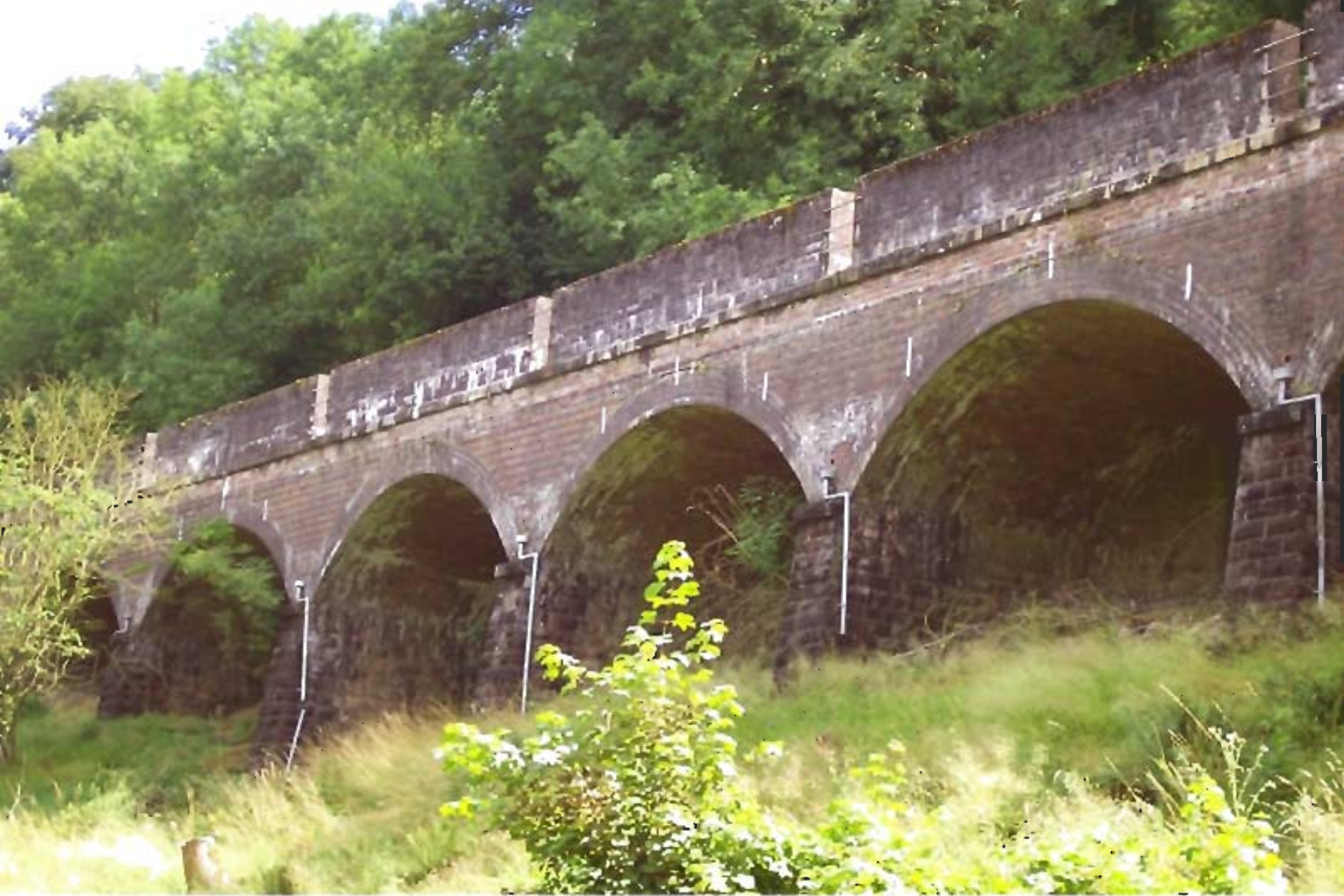
The Slip viaduct (also called Chalford viaduct) This may be considered as a 'half viaduct' as only the 'up' line was on a viaduct and the 'down' line was actually on a shelf carved out of the hillside. The name relates to the fact that a landslip had occurred in the area some years before the railway.
