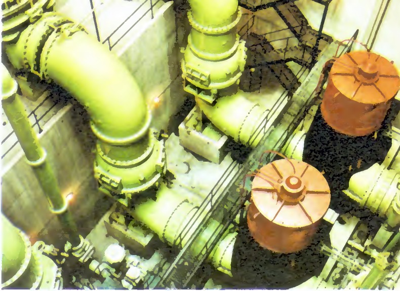
Nos. 1, 2 and 3 circulating water pumps
