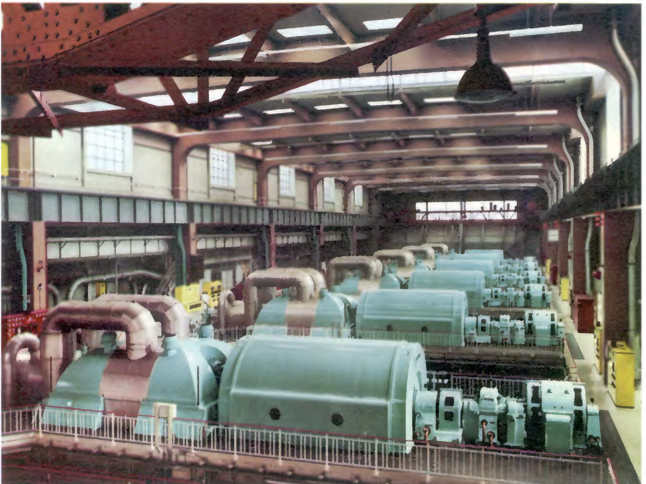
Main turbine hall
