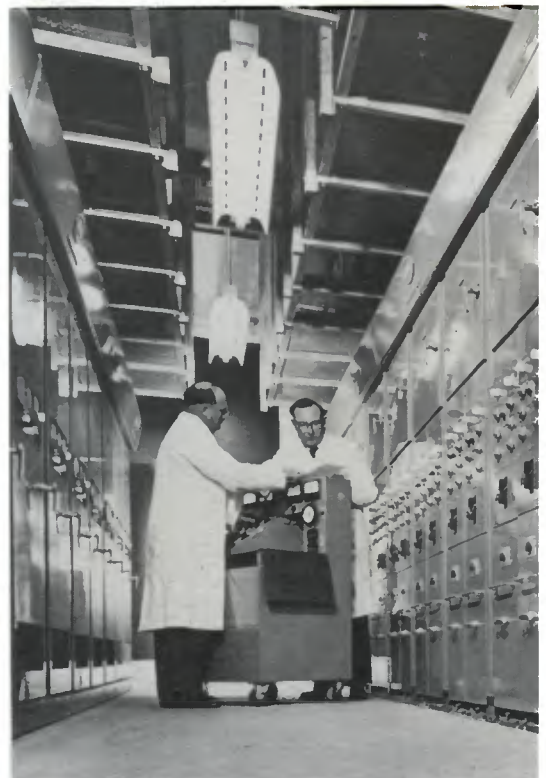
Control rod actuator power unit panels and test trolley
