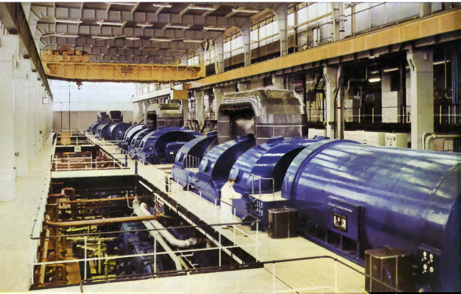
Turbine hall, No. 1. turbo-generator
