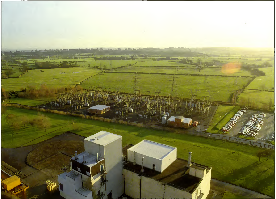
The 132kv grid sub-station.
