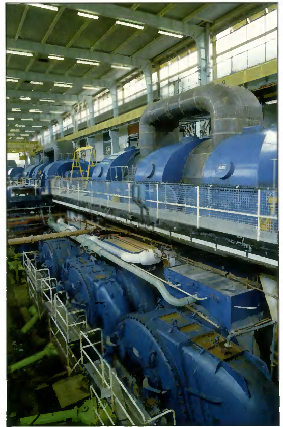
Three condensers are sited under each turbo/generator.
