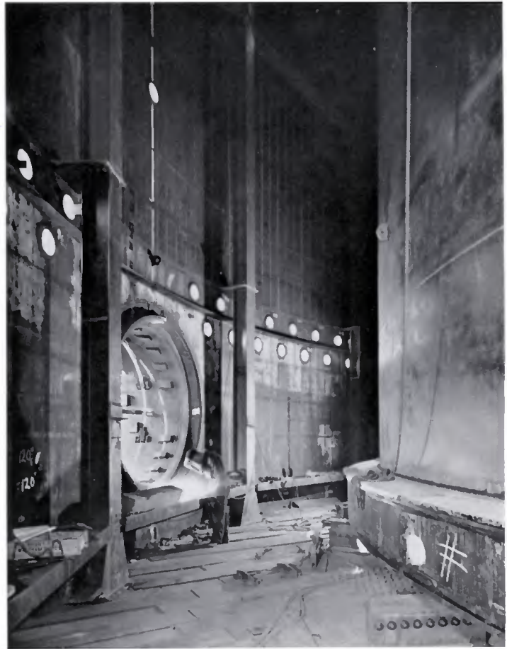
Number 1 reactor—boiler annulus and gas circulator opening
