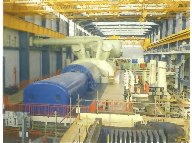
One of the two 313mw turbo/generators.
