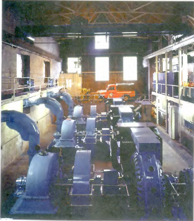
Hydro-electric power: The Turbine hall of the tiny Mary Tavy power station.
